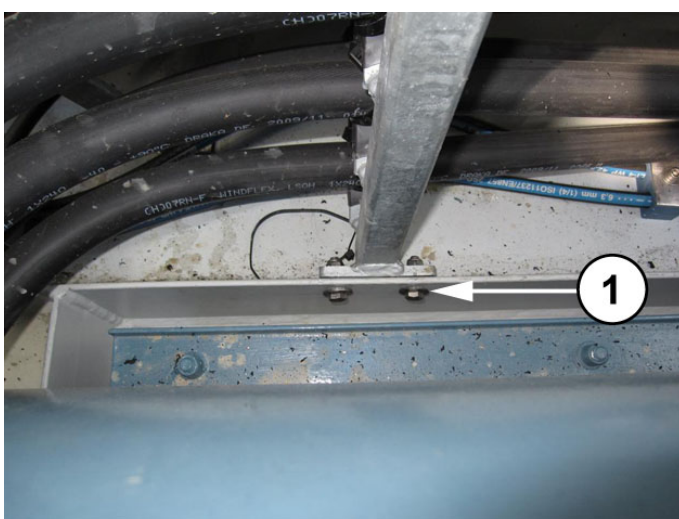
(1) N76 发电机电缆的电缆支架
